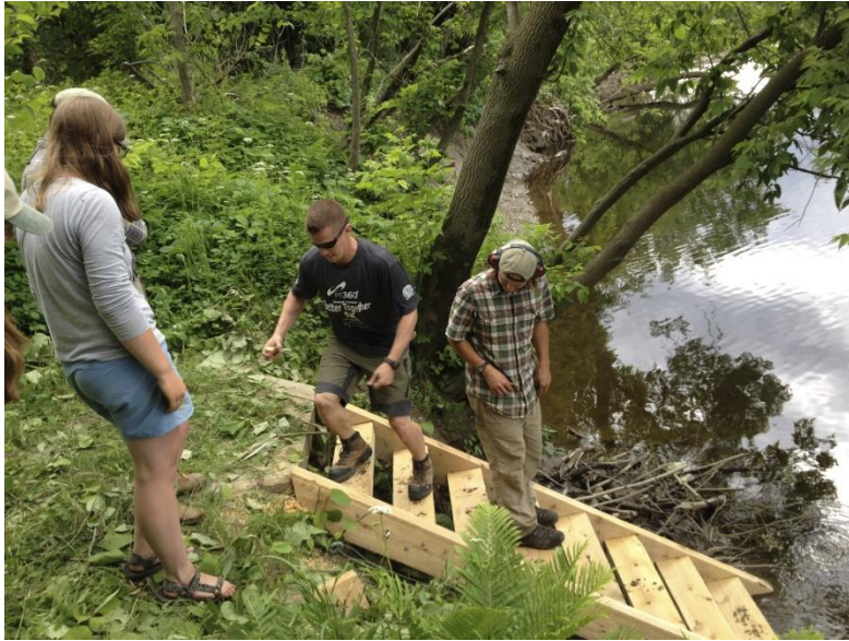
The NFCT Stewardship Crew installs a log ladder to access the Believe It Or Not Campsite.
