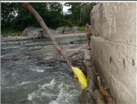
July 2006-A paddler was pinned against the dam remains and pulled below the water and through an undercut hole in the very bottom of the dam. The paddler was flushed by the current to the other side of the dam and received minor injuries.
